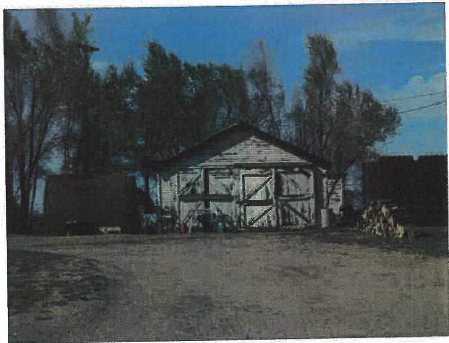
An ancillary structure with deteriorated exterior finishes
