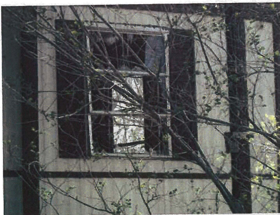
A broken, boarded window
