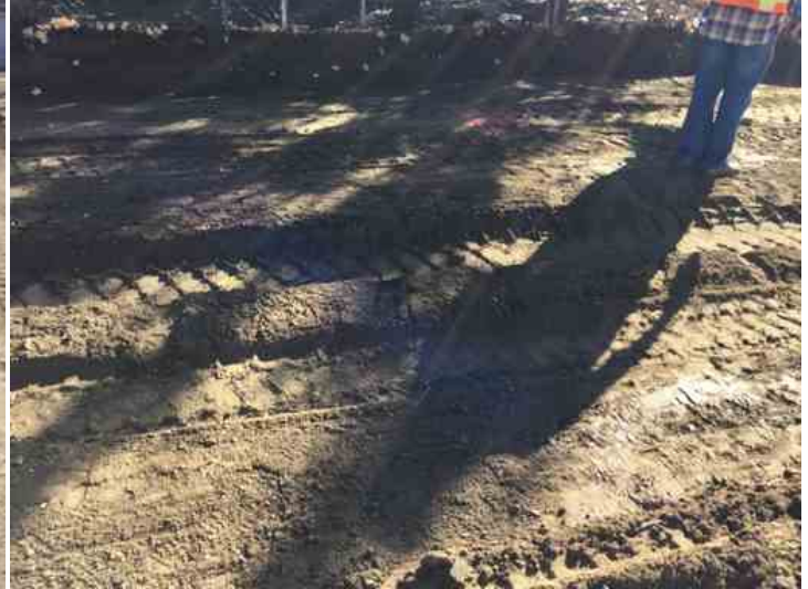
Rutted Subgrade Jackson Drive
