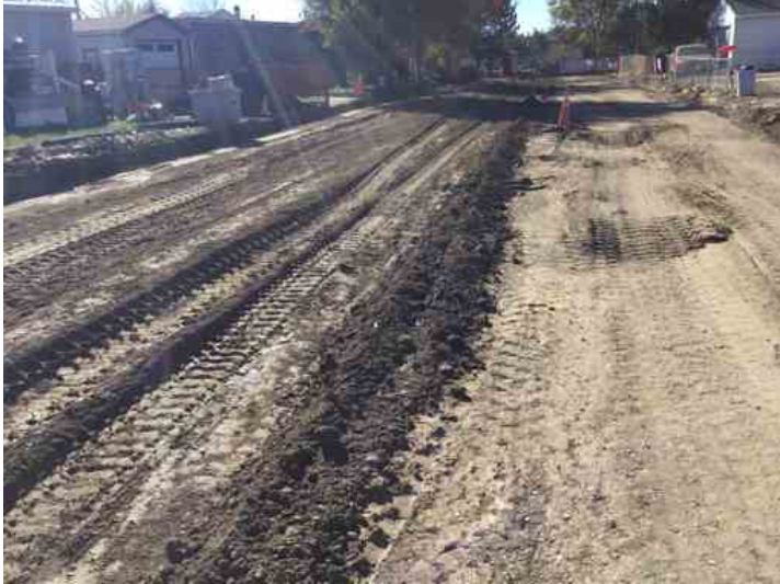
Rutted subgrade at Jackson Drive
